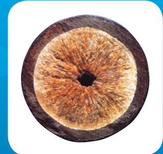
Galvanised pipe heavily scaled
