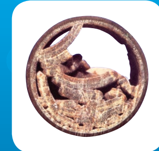
Copper pipe with scale plug
