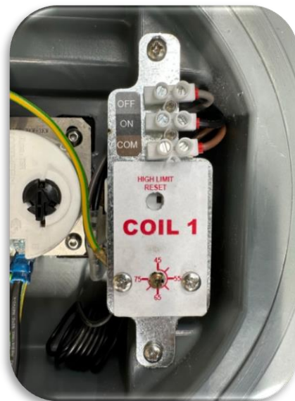
Figure 18 Close up of tank thermostat wiring
