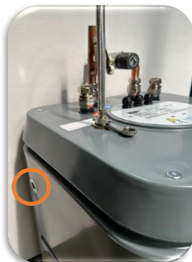
Figure 7 Location of overfill pipe
