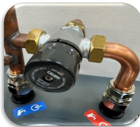
Figure 13 Mixing valve set to position #3
