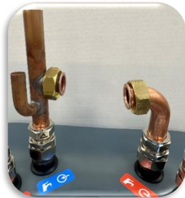
Figure 12 Mixing valve pipe set
