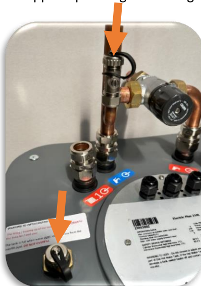
Figure 6 Filling loop disconnected
